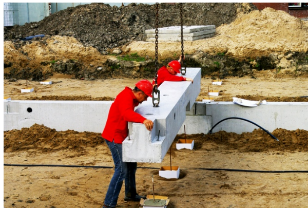
Figure 2e): Plinth beam inserted in the reinforcement slots over the foundation pier.
