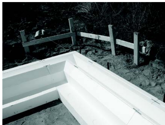
Figure 1a): Prefabricated elements, made of EPS boards glued together and forming an element, are mounted as the strip foundation, fixed together with comb-shaped pieces of plastic.
