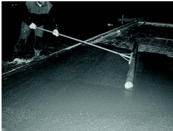
Figure 1c): Iron is mounted, as a net inside the strip foundation and as wires along the moat formed by the two vertical boards of EPS in the prefabricated elements before concrete is cast and levelled.
