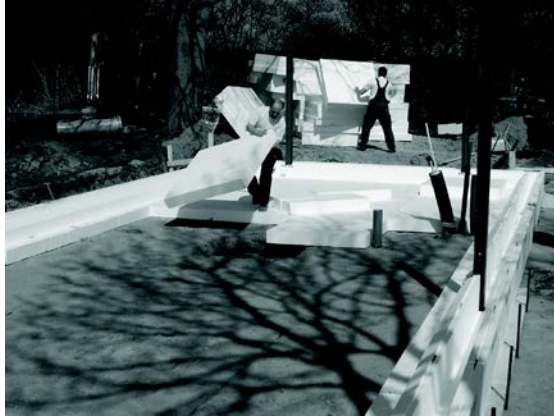
Figure 1b): 300 mm EPS, mounted as two layers on top of the base of stamped gravel bordered by the strip foundation, working as the insulation layer underneath the concrete slab.
