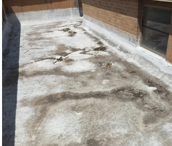
Figure 1: Ponding found during roof inspection.
