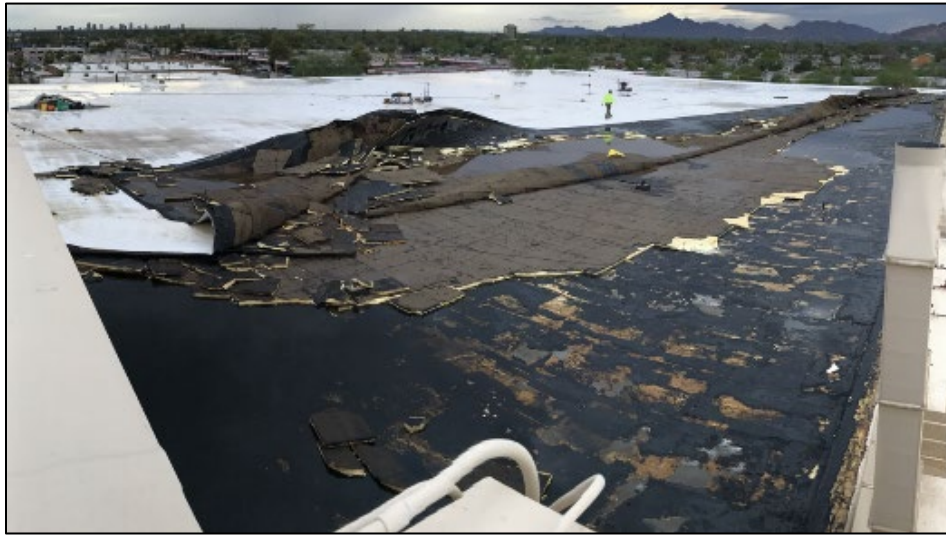
Figure 11: Roof “B” After Storm
